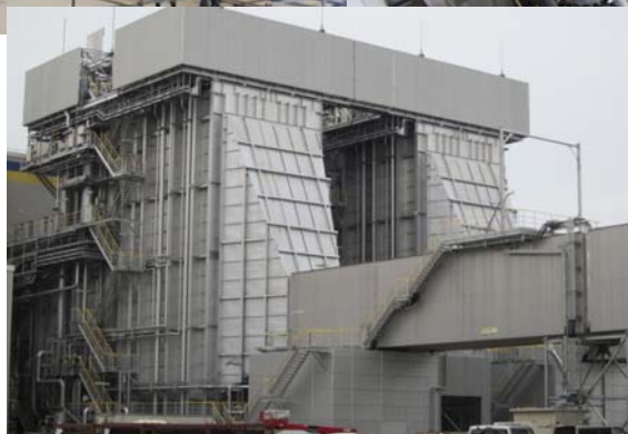
Heat Recovery Steam Generator (HRSG)
