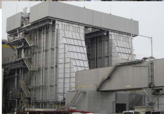
Heat Recovery Steam Generator (HRSG)
