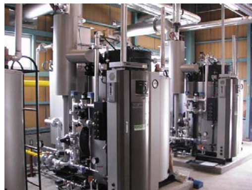
First DME Boiler started commercial operation in 13 th , Jan. 2009
