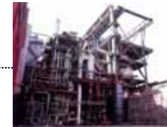
Coke dry quenching equipment (CDQ)
