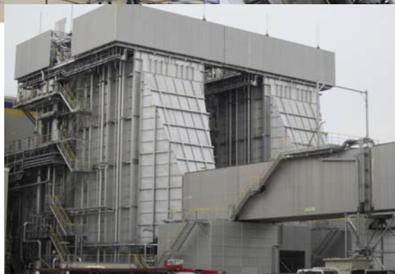
Heat Recovery Steam Generator (HRSG)
